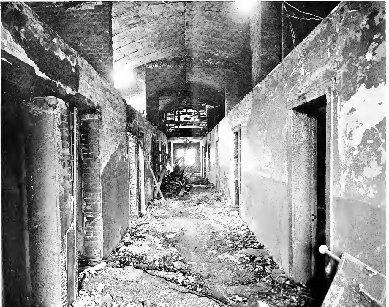
West Wing, Fourth Floor, After the Fire
